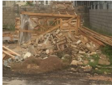
Figure 1. Unsegregated construction waste. Source: Author, 2024.
