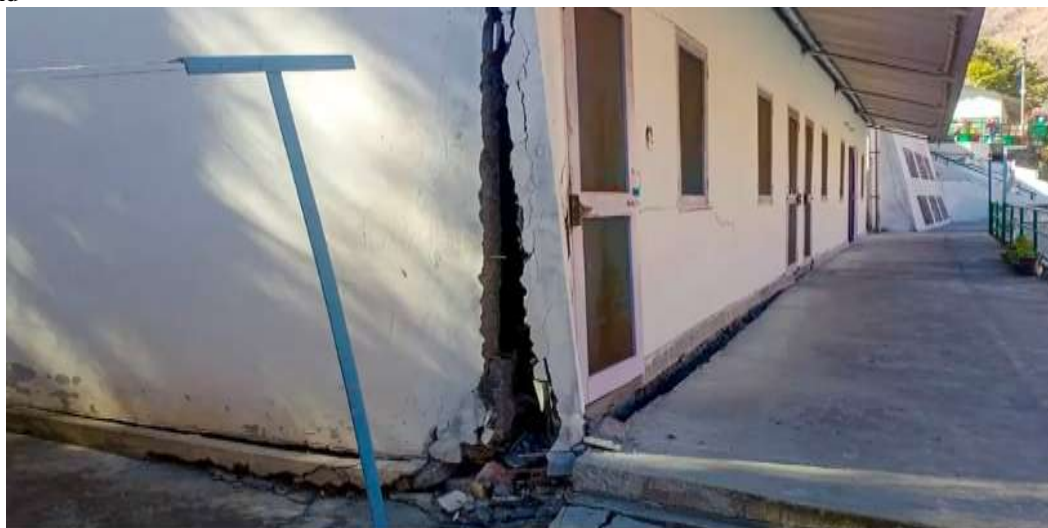
Figure 57 Sinking Town-land subsidence Uttarakhand -widening cracks in houses, roads, collapse January 2023 Reference 49
