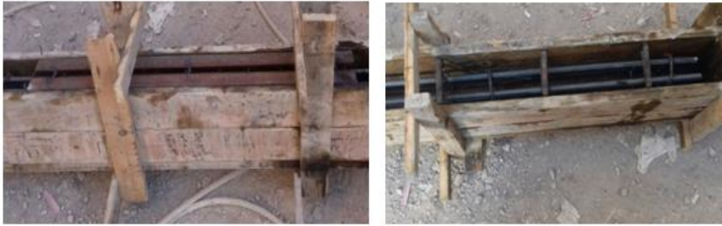
Fig.(7)Welding steel angle in flexure zone Fig.(8)Welding steel plate in flexure zone
