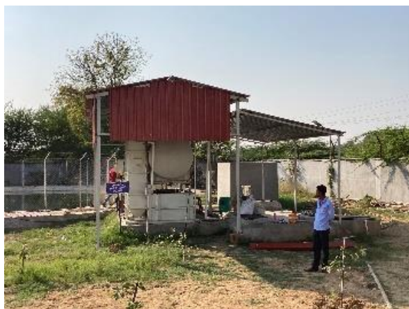
Sewage Treatment Plant & treated water pond
