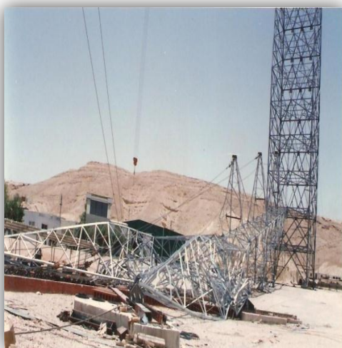
Fig. (3) Test No. (7) 95% Loading Test No. (7) 105% Loading Assumption: (T1) first failure (Destruction Test)
