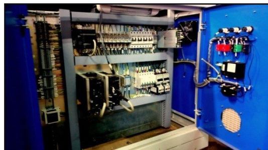
Fig. 5.3 Actual Photograph of Electric Control Panel
