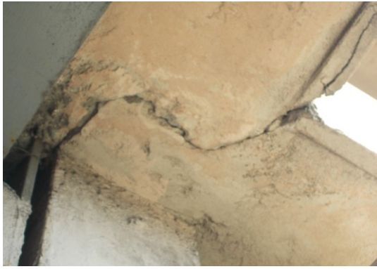
Fig. 3: Cracks at juncture of brickwork & steel column Width: -Below 1mm, Type: -Thin crack, Non-structural Probable causes: - Less bonding between cement and steel, Improper Curing, Shrinkage of slab & thermal variation
