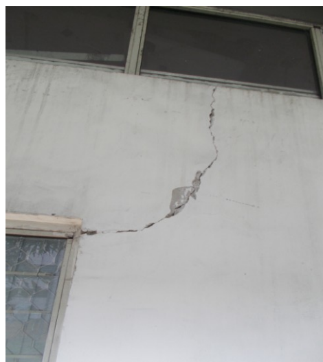
Fig.7: Cracks above window Width: -more than 2mm Type: -Non-structural, Gap crack Probable causes: - Thermal variation, Moisture & Overloading (Kashyzadeh, 1990)
