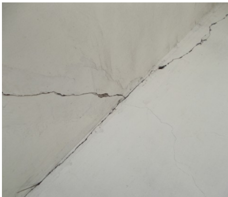
Fig. 5: Cracks at corner of sunshade Width: -Above 5mm, Type: -Gap crack Probable causes: - Improper cantilevering, Due to joint, & Heavy exposure to water
