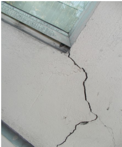
Fig. 1: Cracks below window sill level
