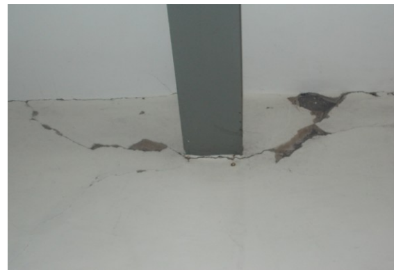
Fig. 6: Cracks below a beam Width: -Above 2mm Type: -Structural, Medium cracks Probable causes: - Due to Overloading, & Improper Design
