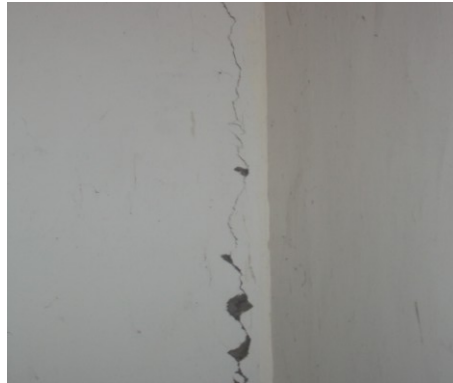
Fig. 4: Vertical cracks in wall Width: -Between 1mm to 2mm Type: -Non-structural, Medium Probable causes: - Temperature Variation, Shrinkage, & Moisture Changes
