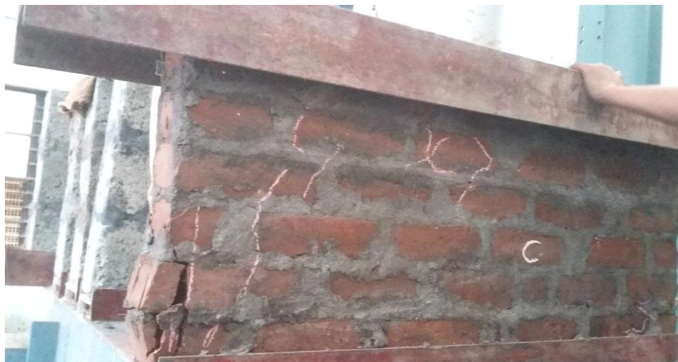
Fig4: Failure pattern of Brick wall
