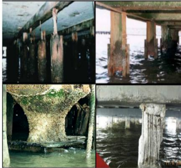
Figure 13: Degradation of traditional piles
