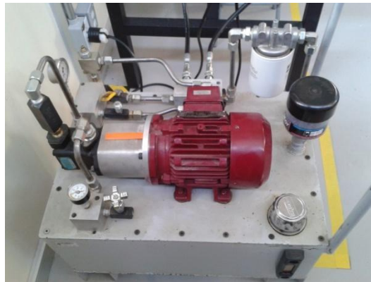
Figure 9. Hydraulic Power Unit.
