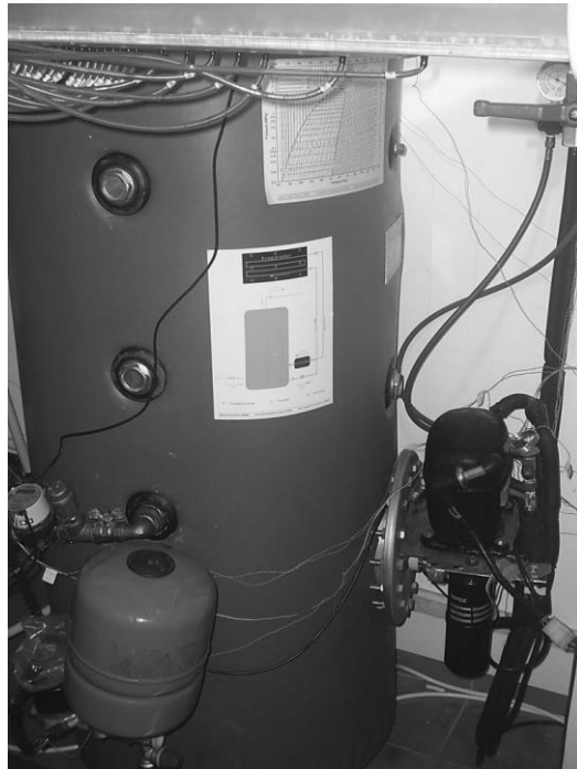
Fig. 2. Thermal storage tank and compressor
