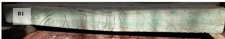
Figure 3: Crack pattern of MK_0S_1A_1C_1B
