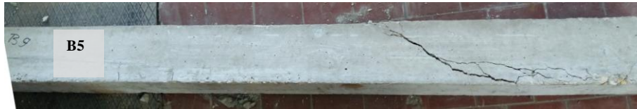
Figure 7: Crack pattern of MK_1S_3A_1C_1B
