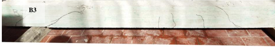
Figure 5: Crack pattern of MK_1S_1A_1C_2B
