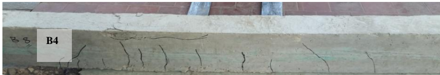
Figure 6: Crack pattern of MK_1S_2A_1C_1B
