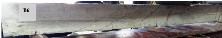
Figure 8: Crack pattern of MK_1S_1A_2C_1B
