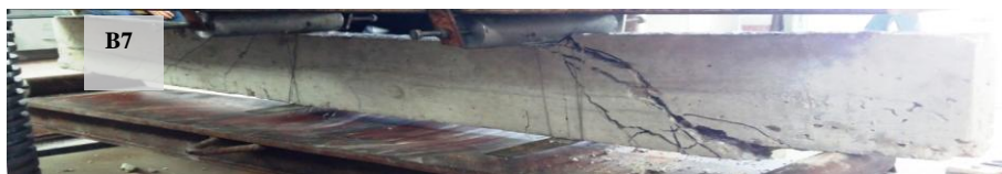
Figure 9: Crack pattern of MK_1S_1A_3C_1B
