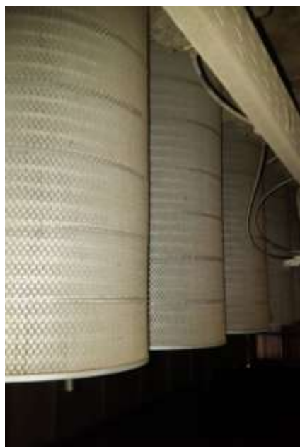
Figure 1. Filter Air Intake GT 13E2
