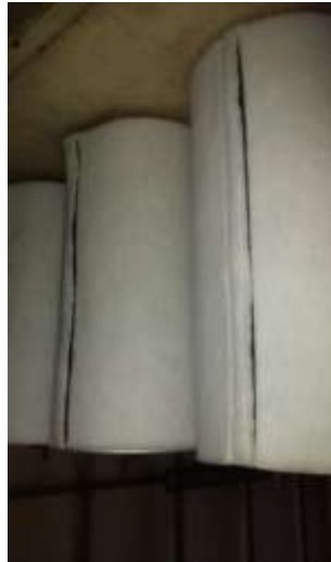
Figure 10. Prefilter in Filter Air Intake
