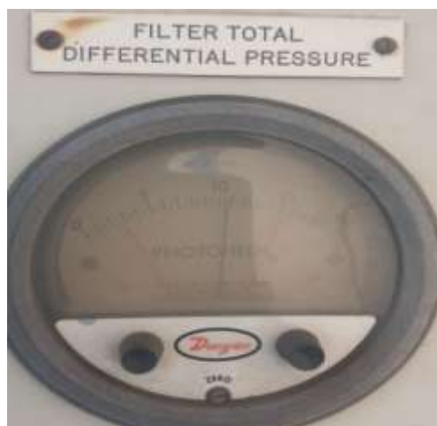
Figure 6. Dp Air Intake GT 1.2 Indicator
