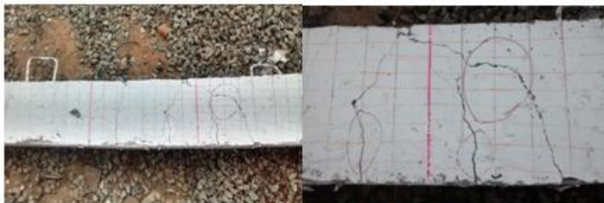
Fig.8 cracking pattern of beams
