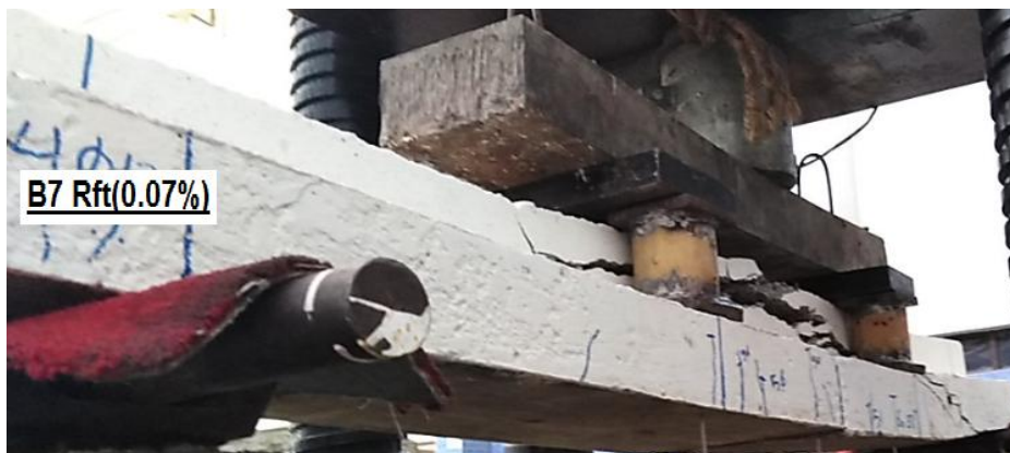
Figure (14): Crack pattern for control beam (B7)
