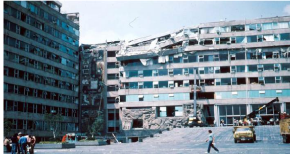
Fig. 1: Damage to Reentrant corner and upper stories of the Ministry of Telecommunications Building in Mexico City after the 1985 earthquake.
