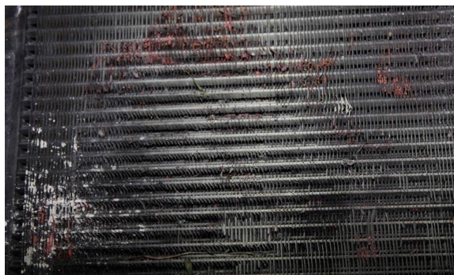
Figure 5: Damaged radiator due to using surface water
