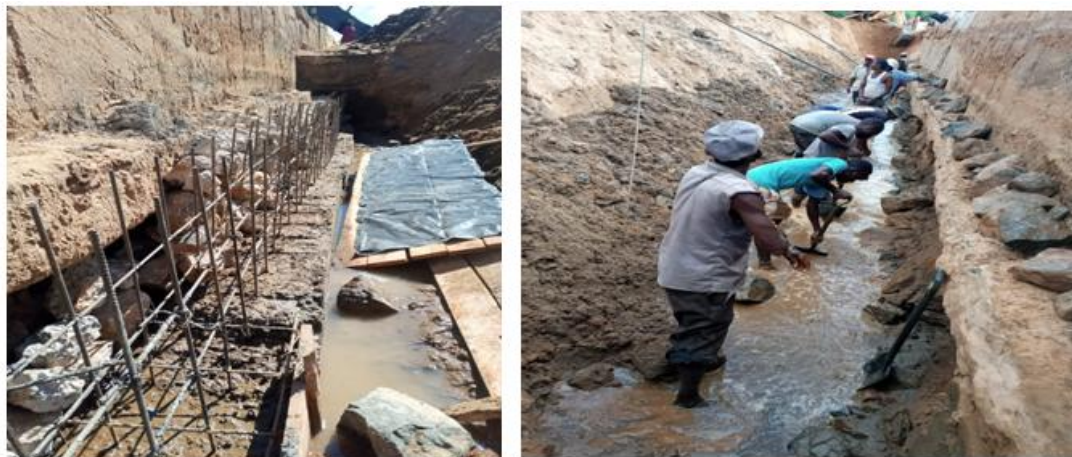
Plate 1.4: Enziu River at Kurura showing foundation of the wall not properly anchored to stable ground causing under foundation seepage of water. Improved Engineering correction to control seepage.
