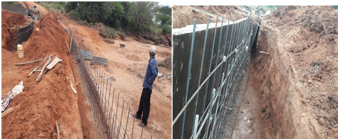
Plate 1.2: shows construction of a level drift which acts as an access through the river and at the same time acts as sand dams at Katilini in Kitui South.
