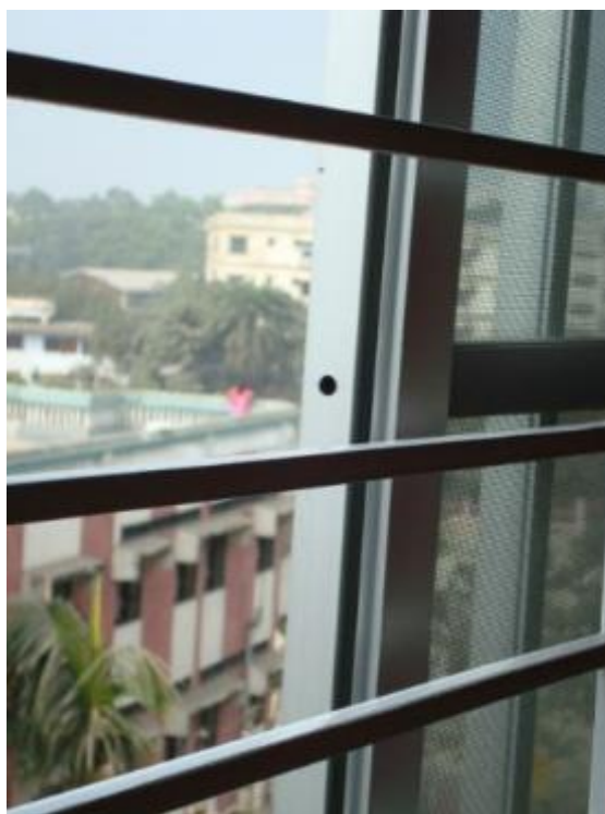
Figure 12: Typical photo of window (Tahmina, 2009).
