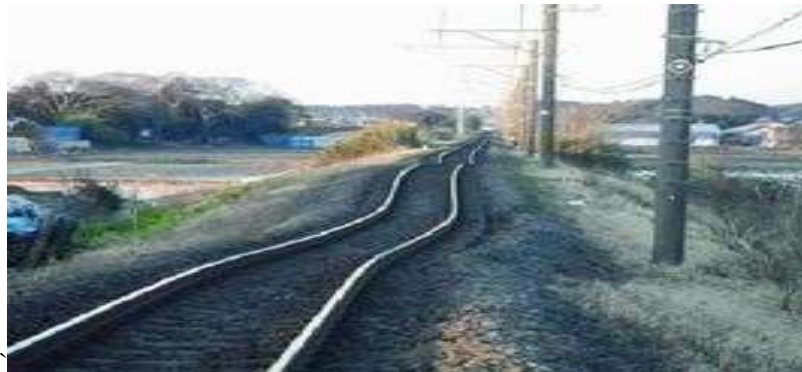
Figure 6 Track settles differentially
