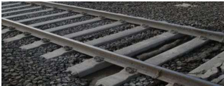
Figure 2 Track fouls due to mud pumping
