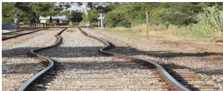
Figure 3 Track buckles due to lack confining pressures
