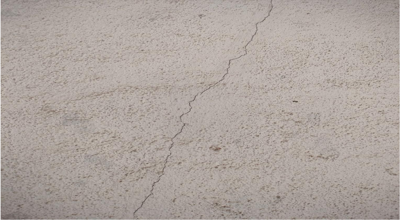
Fig.No.4.7 Load bearing wall (Damaged State)
